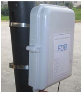
FDB fiber termination box on the pole
