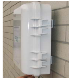
FDB fiber termination box on the wall
